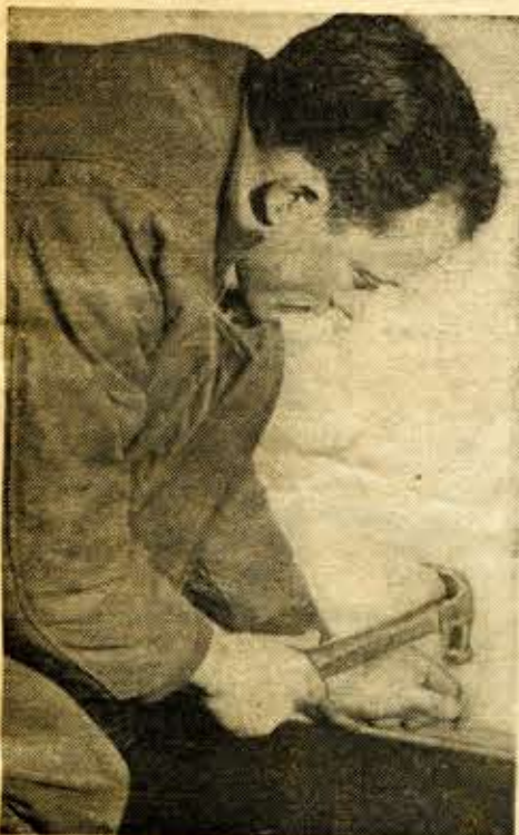
Joe Johnson, carpentry instructor at the Salt Lake Area Vocational School, shows how flooring next to a wall may be surface nailed.
