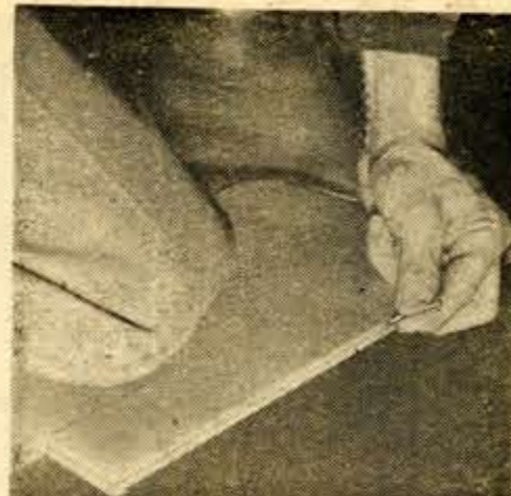
Here's how the flooring is nailed—at an angle of 50 degrees and through the angle of tongue. Use firm strokes.
