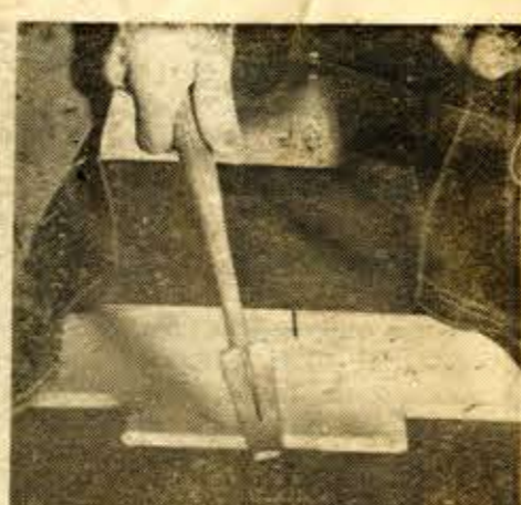
If the boards are sprung, you can straighten them in place by using a scrap piece as a pouncing block.
